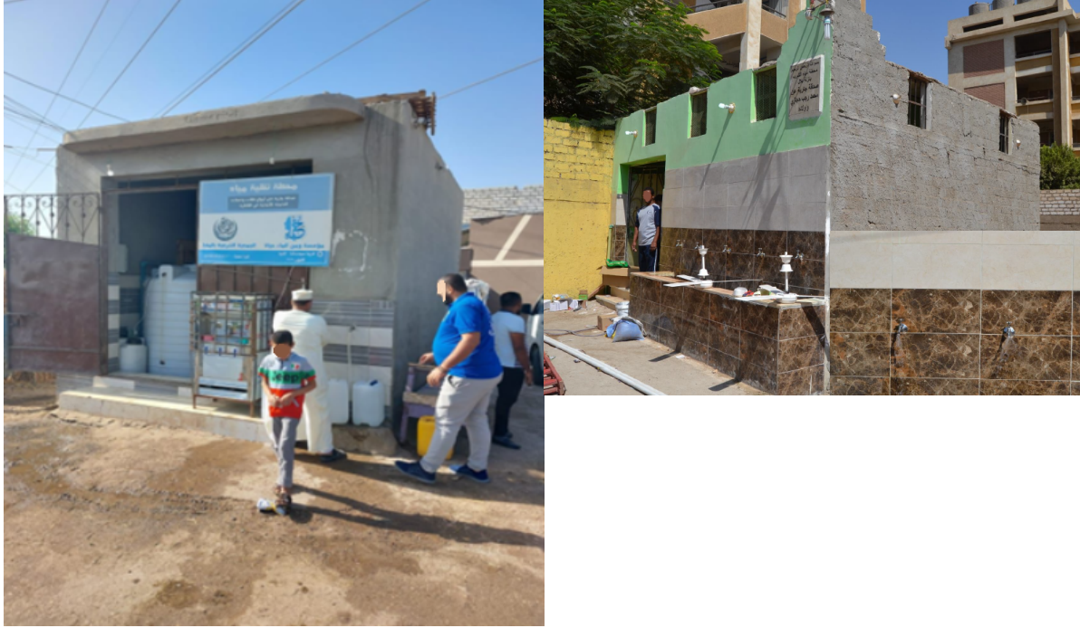
Figure B1. Water Treatment Units
